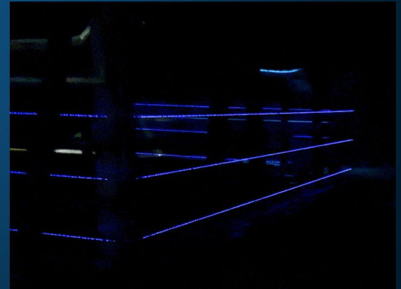
Corona discharge during operation
