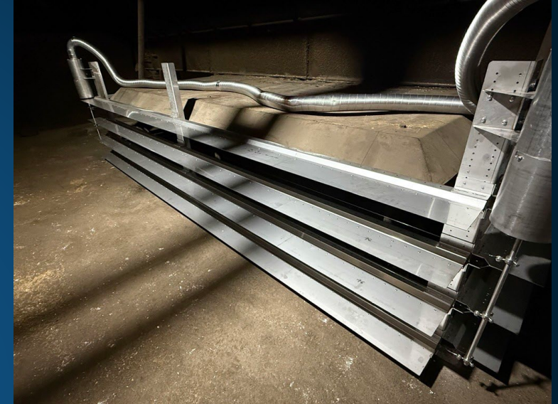
ESP installation below kiln inlet
